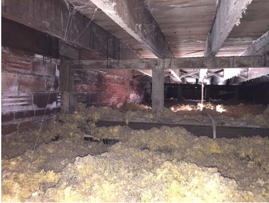
View of roof structure and wood construction on top of steel beam
