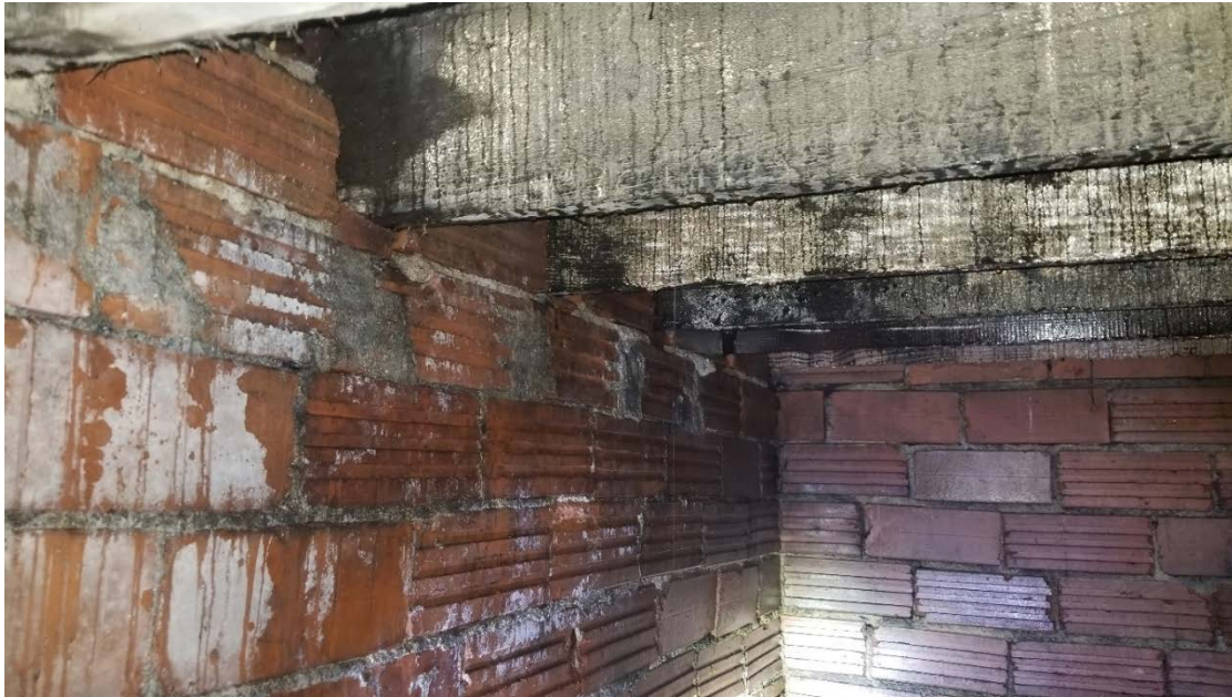
View from inside attic space of northeast corner showing joist bearing on clay tile wall
